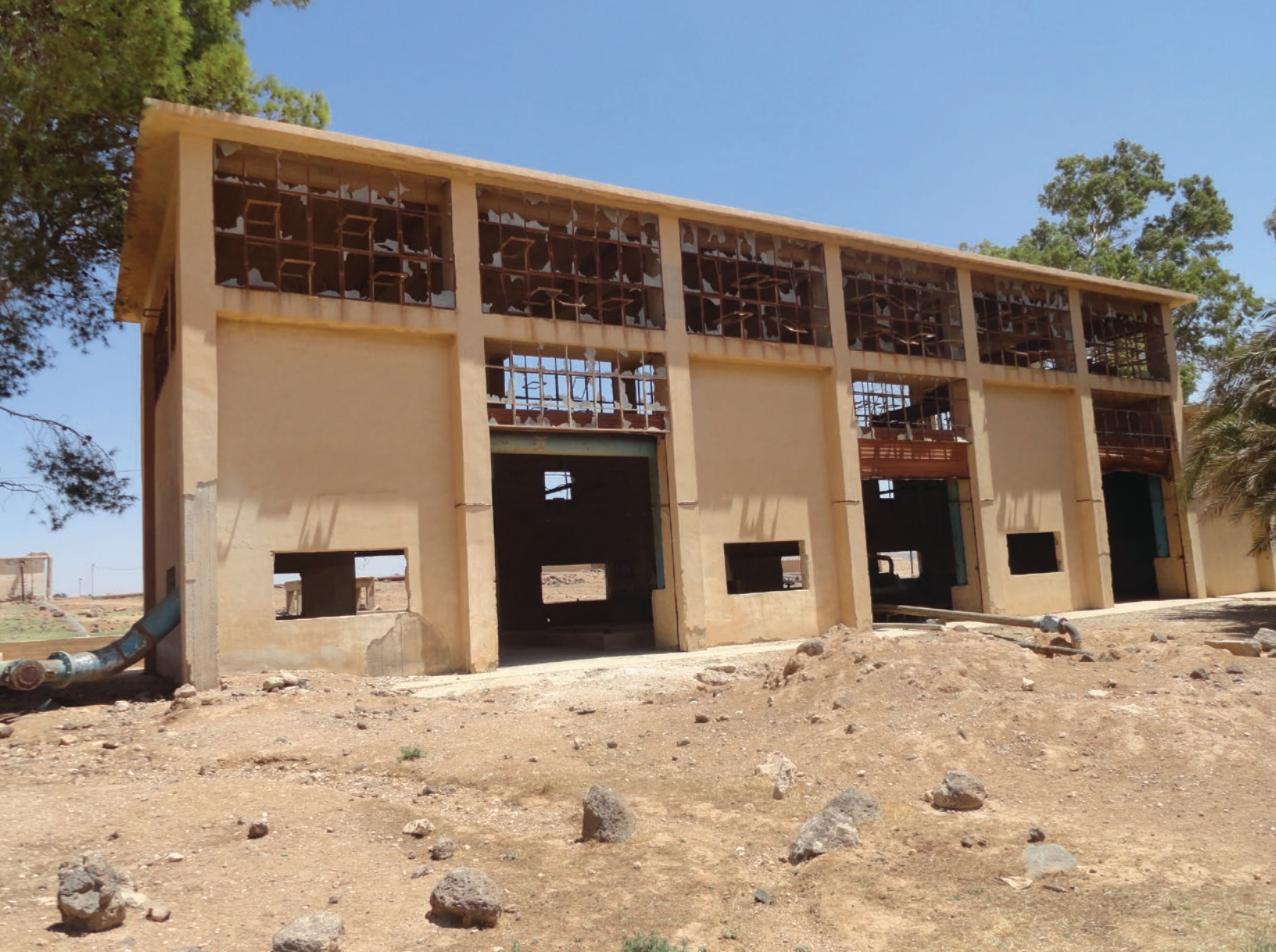
Beshriyyeh Pumping Station located east of Mafraq city in Jordan before being rehabilitated by the ICRC in support of the Yarmouk Water Company, August 2016. The station serves more than 11,500 Jordanian residents and Syrian refugees. © A. Otoom/ICRC.
