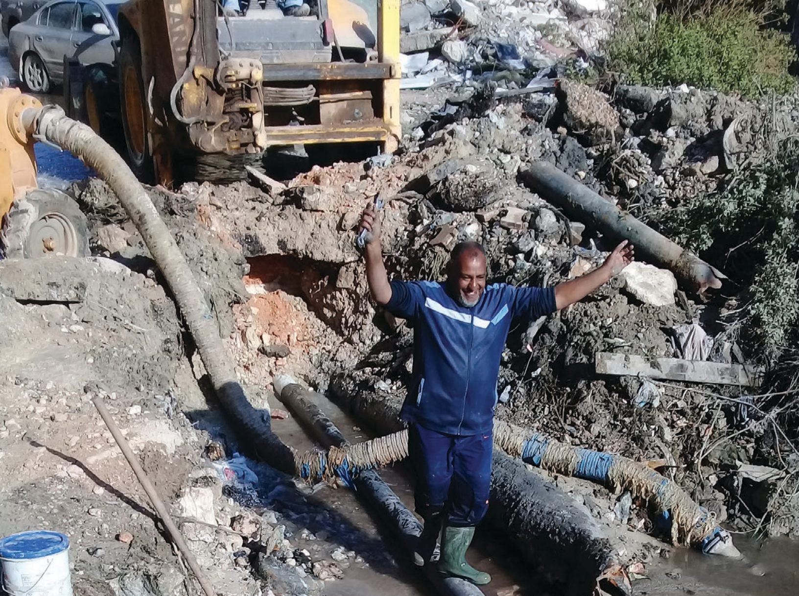
Water authority technician celebrating the end of maintenance works on one of the main water pipelines affected by the hostilities in Benghazi downtown, 2018. © A. Albarasy/General Company for Water and Wastewater (Libya).
