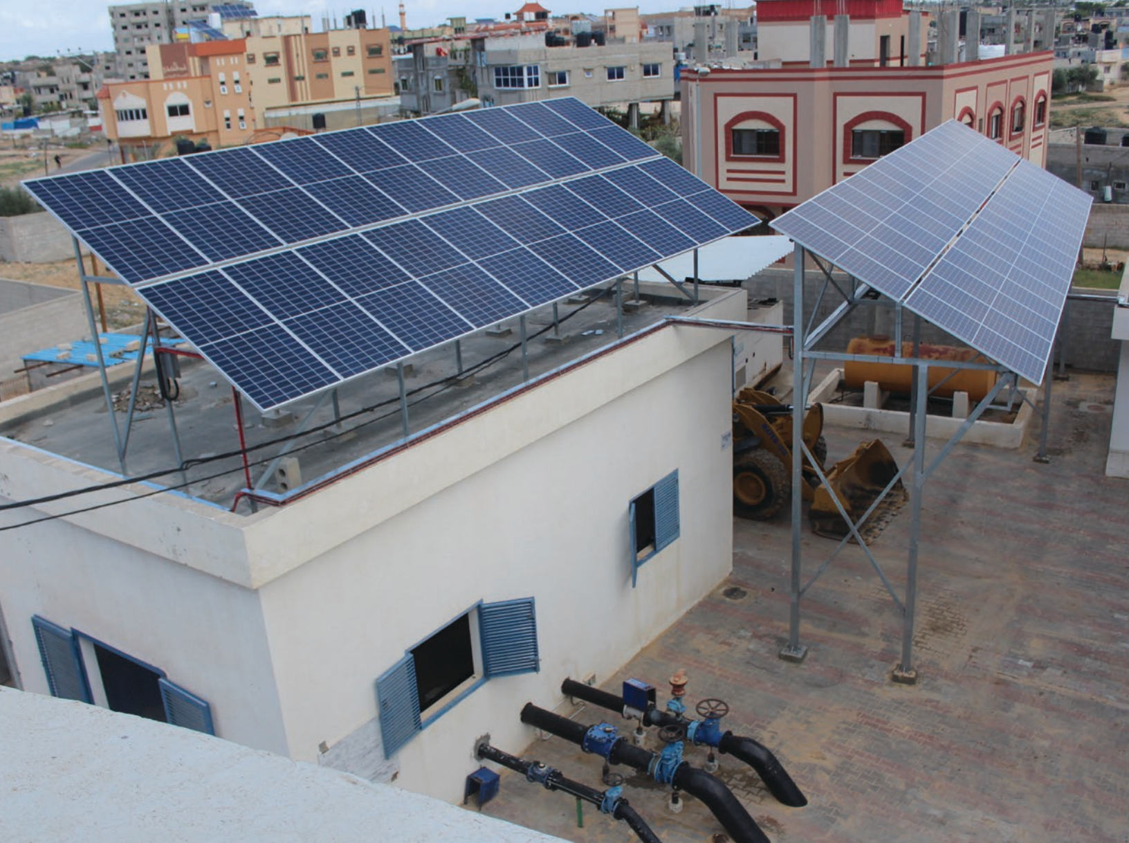
Canada Well, Rafah, Gaza, 2019 - In support of the Coastal Municipalities Water Utility, the ICRC installed Solar PV, a net metering system, and a dedicated power line to improve the operational resilience in water supply and reduce operating costs for a critical public water supply facility. © H. Mhanna/ICRC.
