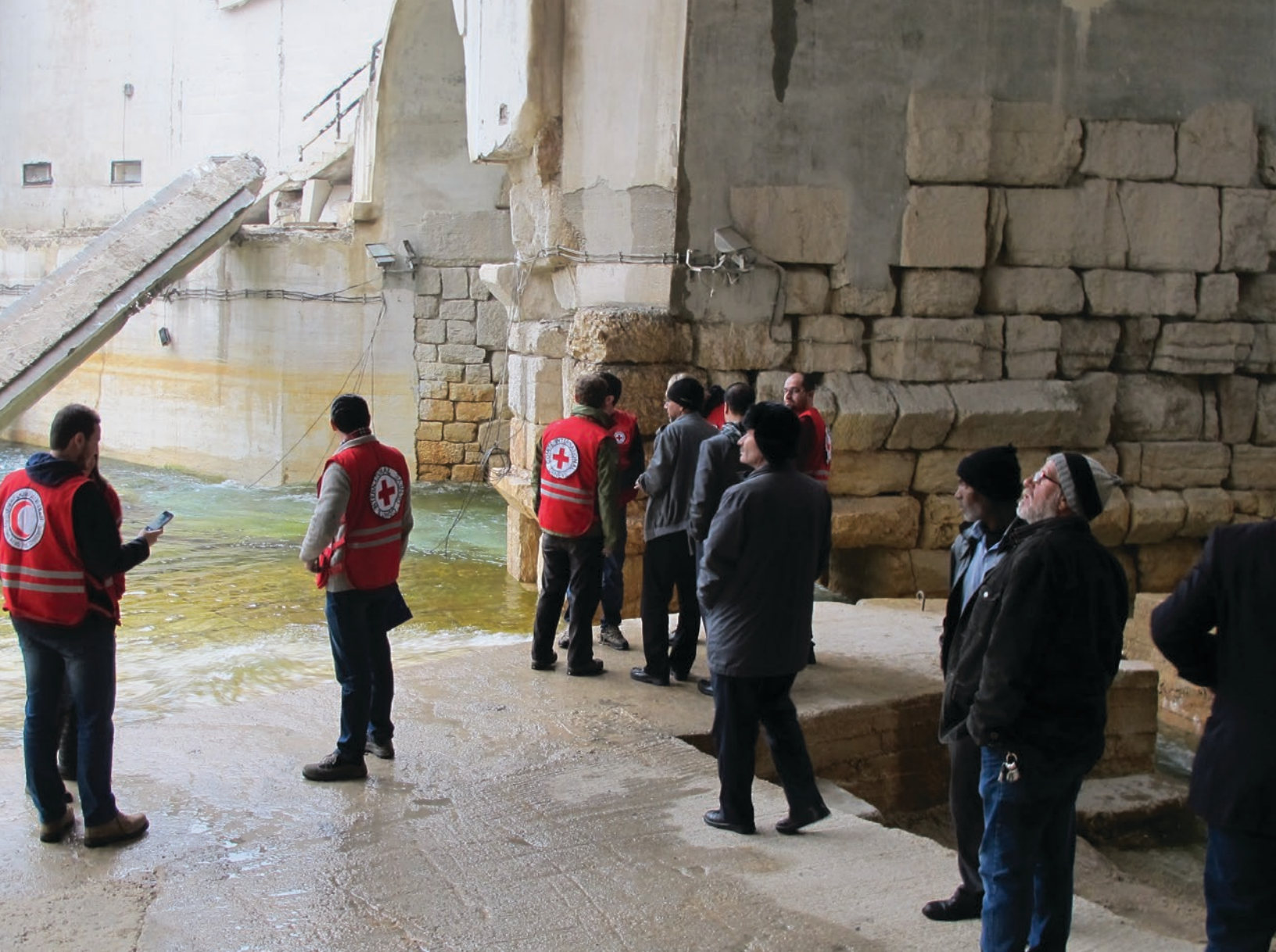
Assessment visit to the damaged Fiegh Spring catchment; the main drinking water supply source for the city of Damascus and some surroundings, from which approximately 5,000,000 Syrian residents and internally displaced people benefited. © L. Khalil/ICRC.
