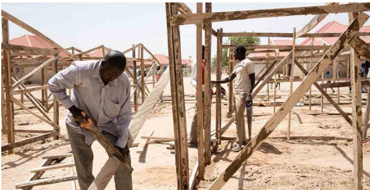
Nigeria, Gubio camp. The ICRC is supporting the construction of shelters for newly displaced people.
