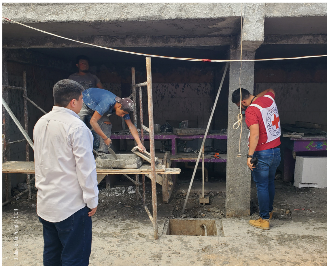
In Veracruz, we supported the Las Patronas collective by remodelling the roof of their dining room, thus helping them have adequate infrastructure for providing food services to migrants.
